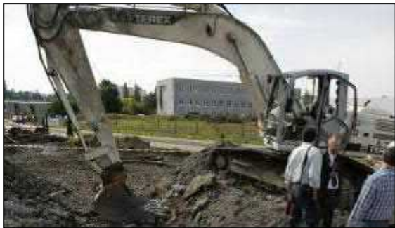
WWII bomb injures 17 at construction site in Hattingen, Germany – 2008.
